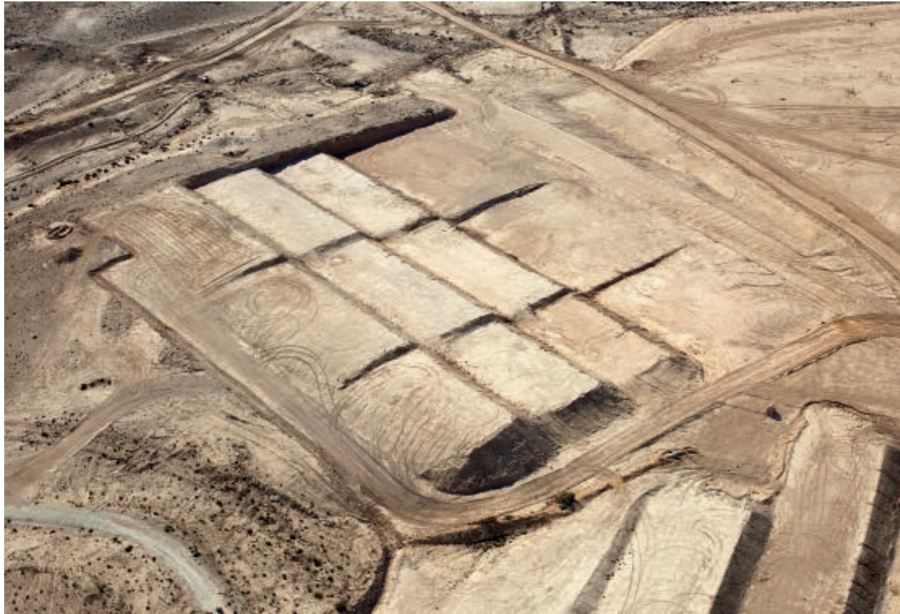
EARTHWORKS FOR 'IR HABAHADIM (CITY OF MILITARY TRAINING BASES), &lt;100 MM RPA
